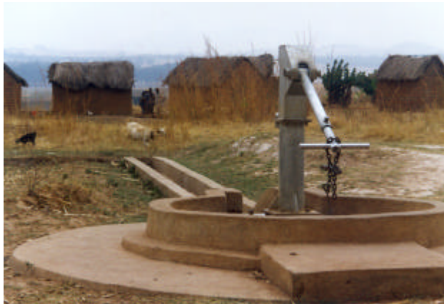
A community administered water pump in Caala, Huambo, organised by Development Workshop
