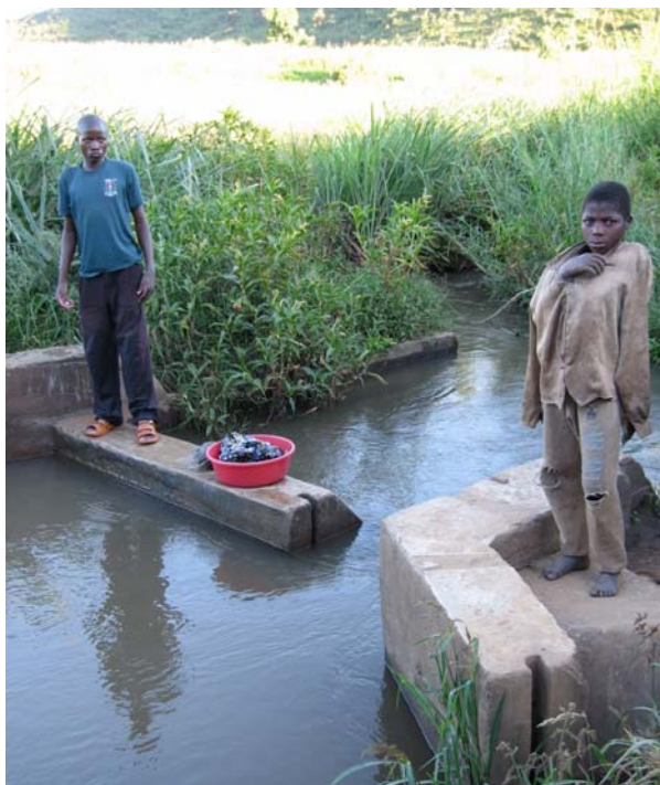
The intake for the Msanzi irrigation scheme: the gates for diverting water no longer function
