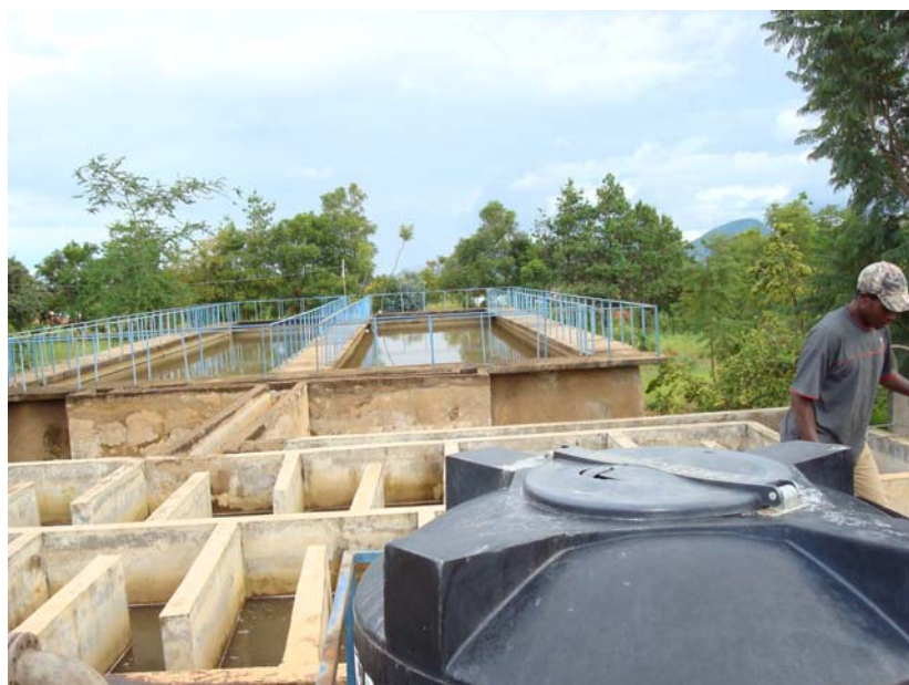
The sedimentation tank for Sumbawanga town water supply started as a “joint venture” with RUDEP in 1995 but was not officially opened until 2006
