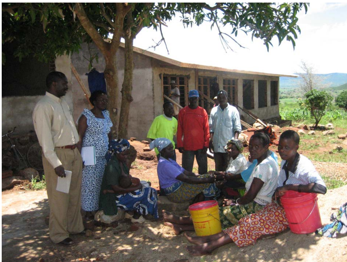
Photo 2. Women in Ileje doing ‘voluntary’ work for the construction of a secondary school. The male hamlet leader to the left is organising the women’s work. Pregnant women who have registered their pregnancy are exempted from this kind of work (by Siri Lange).
